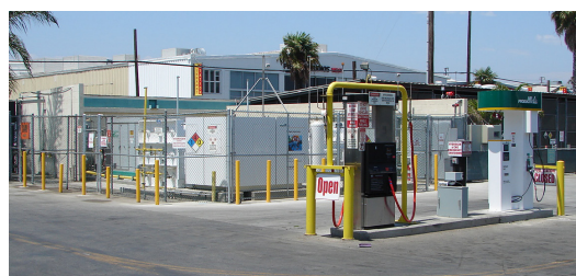
Figure 2: Hydrogen station at the City of Santa Monica fleet yard in 2006
